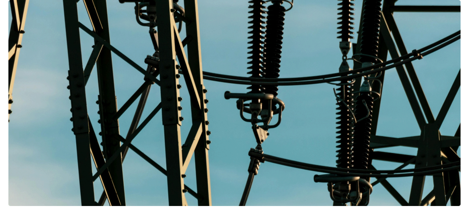
Power infrastructure — Crown Mountain core supply focus
